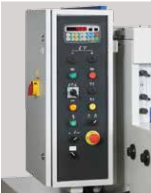
Control panel and electrical circuit in the same cabinet for easy reach
