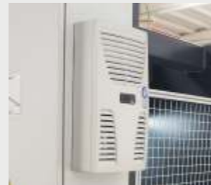
Electrical Cabinet Cooling System
