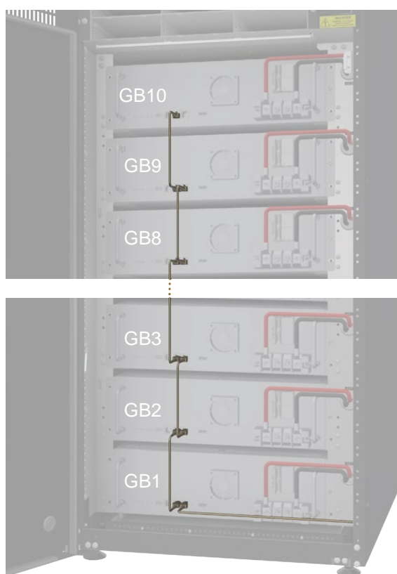
Figure 4.22 Battery communication cables
